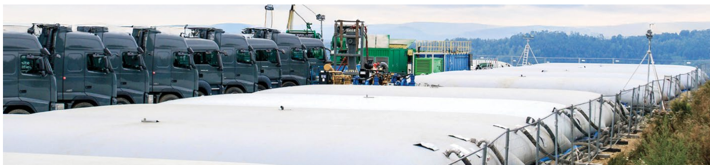
Mobile water base with a capacity of 3000 m 3 .
